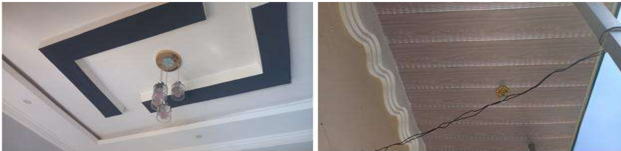
Figure 16: Ceiling Condition at FSTP Site
