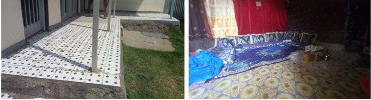
Figure 15: Floor Condition at FSTP Site
