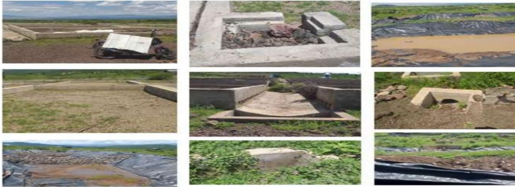
Figure 3 Partial view of Existing drying beds structural problems AMT
