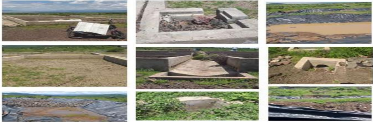
Figure 2: Partial View of Existing Drying Beds Structural Problems AMT, Photo by the Consultant
